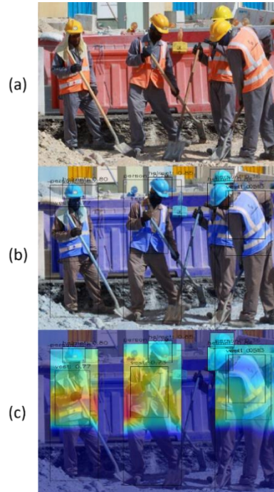
Figure 37: (a) Initial image for Construction Safety Measures (b) Detected Safety Objects (c) Eigen-CAM Safety Objects Analysis
